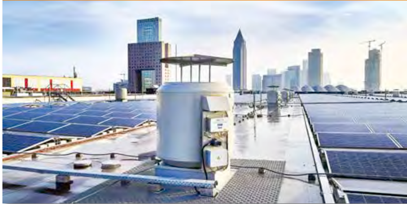
On the roof of Hall 12: TROX X-FANS smoke exhaust fans of Type BVD, fitted with the intelligent fan diagnosis system.
