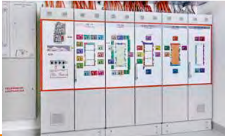
Proven and reliable systems: The fire alarm system has pictures of the hall as well as colour diagrams of various scenarios. This helps the fire brigade to immediately see where an incident has happened. With manual push buttons they can quickly initiate the correct actions.
